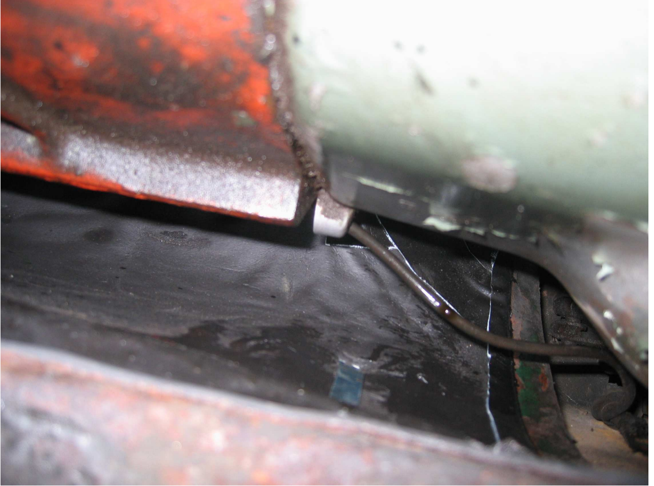
Picture #4 - Here is an underside picture of the tunnel in place. It does cut down on the sound / heat. All the best for the trail, Mark Buggy
