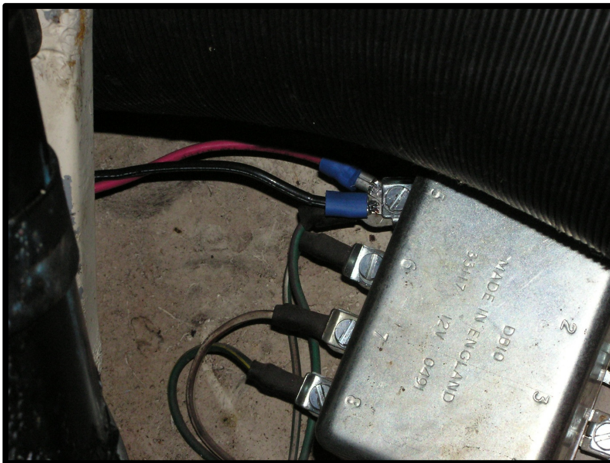
Close up of the relay box showing the Red wire from the Third Brake Light and the Black wire from the Mechanical Brake Light Switch attached to Terminal 5. I used Ring clips for security. Colors vary to indicate the circuit.
