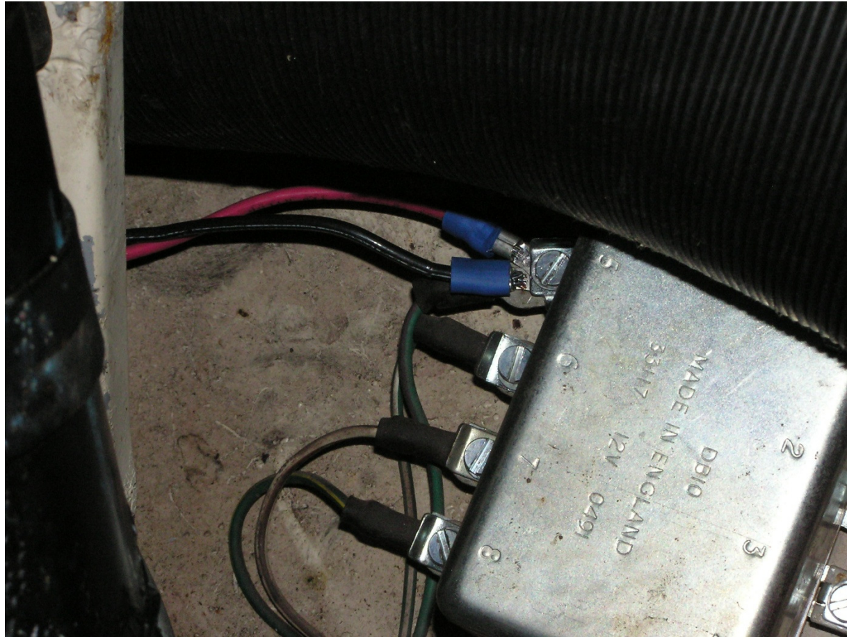
Close up of the relay box showing the Red wire from the Third Brake Light and the Black wire from the Mechanical Brake Light Switch attached to Terminal 5. I used Ring clips for security. Colors vary to indicate the circuit.
